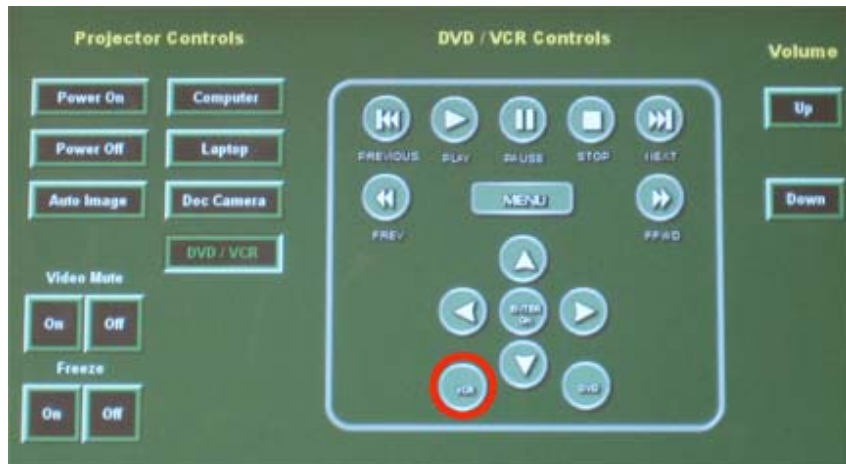
FIGURE 7 ("VCR" button on AMX touch screen switcher)
